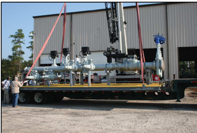
Ultrasonic Metering Skid
